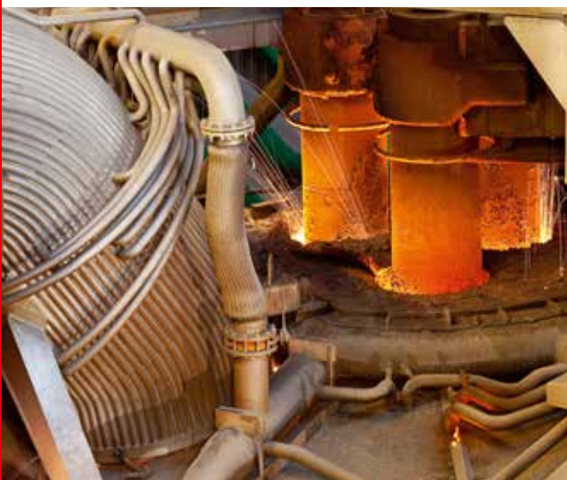
ARCESS® electric arc furnace with a tapping weight of 135 tons.
